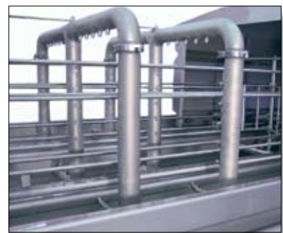
Tunnel Washer spray manifolds
